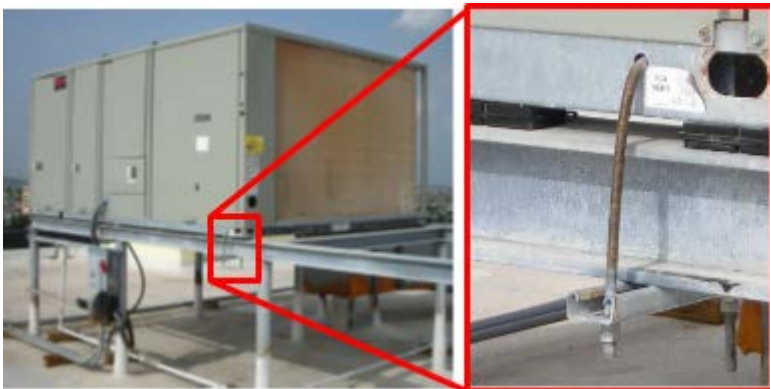
Example of large equipment with non-engineered connection
