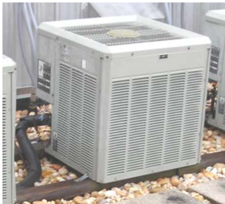
Limited attachment to unsecured wood blocking
