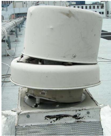
Wind damage to fan cowling Photo source: FEMA
