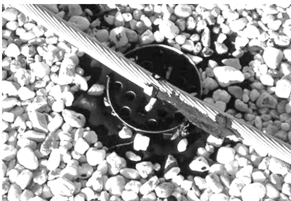
Conductor secured with clip adhered to roof cover
