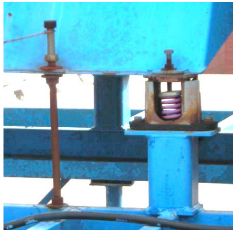
Vibration isolator with threaded rod for upward travel limit Photo source: Rich Gallagher, The Zurich Services Corporation
