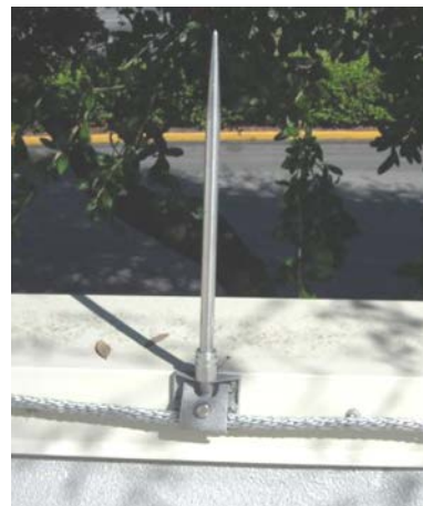
Air terminal screwed to wood nailer
