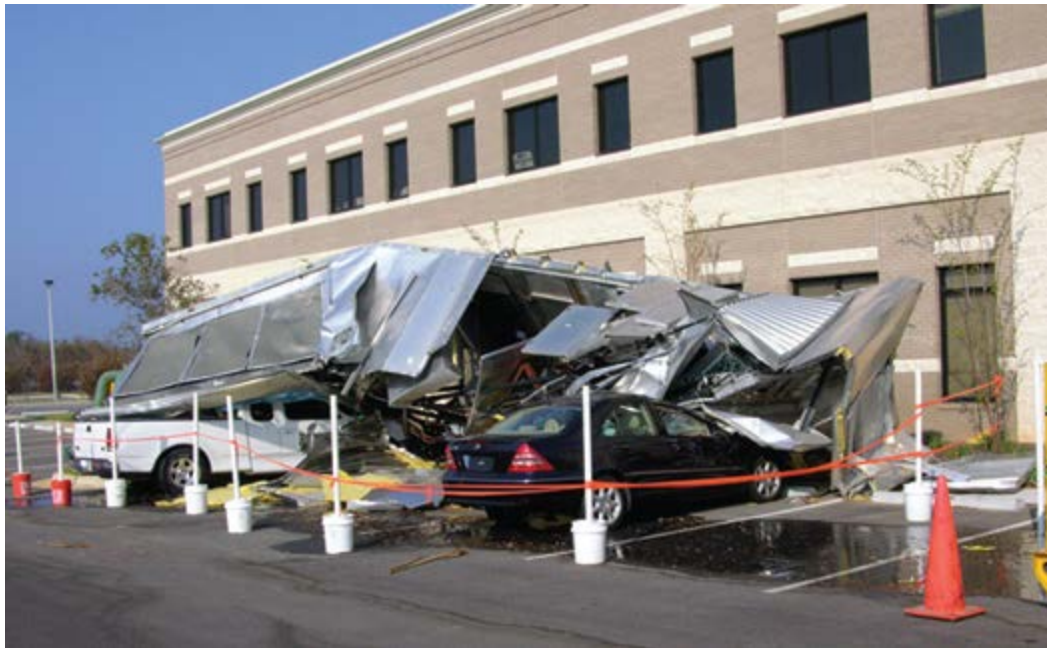
Per the FEMA guide (see Reference 3) "Attachment of Rooftop Equipment in High-Wind Regions", this 18,000 lb. HVAC unit was secured to curb with 16 straps with only one screw per strap. An estimated wind speed between 85-90 mph dislodged this unit from the roof. Photo source: FEMA
