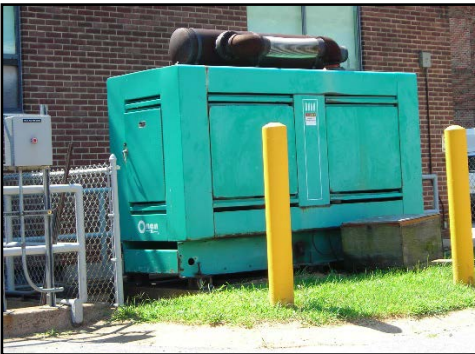
Bollards provided to protect emergency generator from physical injury
