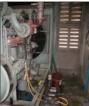
Combustion air louvers that allow carry-over of wind-driven rain
