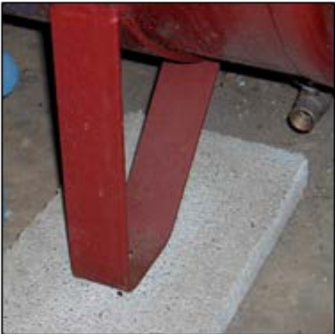
Fuel tank leg not bolted to floor
