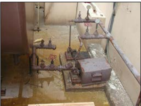
Fuel oil pumps within dike area of outside main fuel tank
