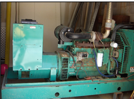
Diesel engine driven emergency generator
