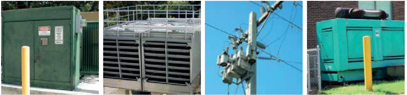
Transformer, generator, cooling tower, and overhead wires (Photo source: Rich Gallagher, The Zurich Services Corporation)
