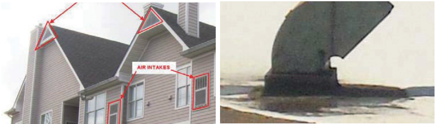
Left: Building wall openings (Photo source: Sam Goddard, The Zurich Services Corporation)
